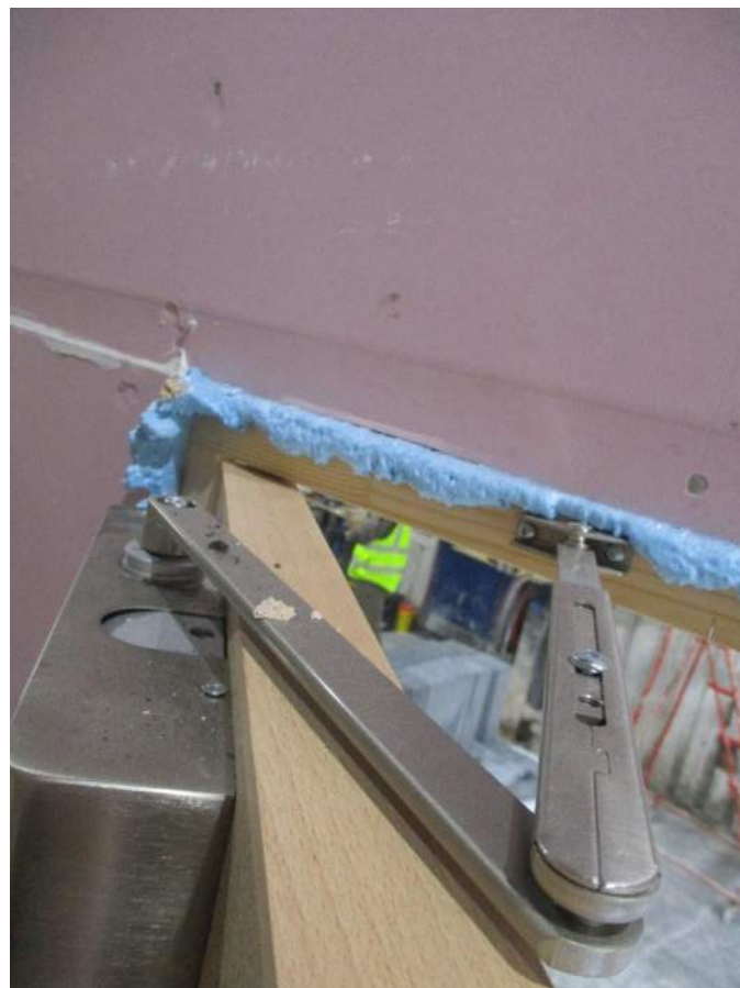
Figure 29 Closer – Both Doorsets
