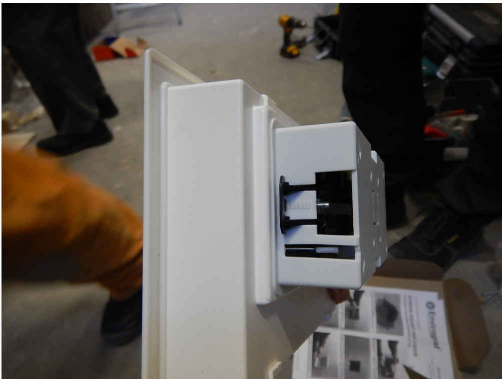
Foto C.4 Detail of the Sunken Socket and back box with two gang socket facia assembly
